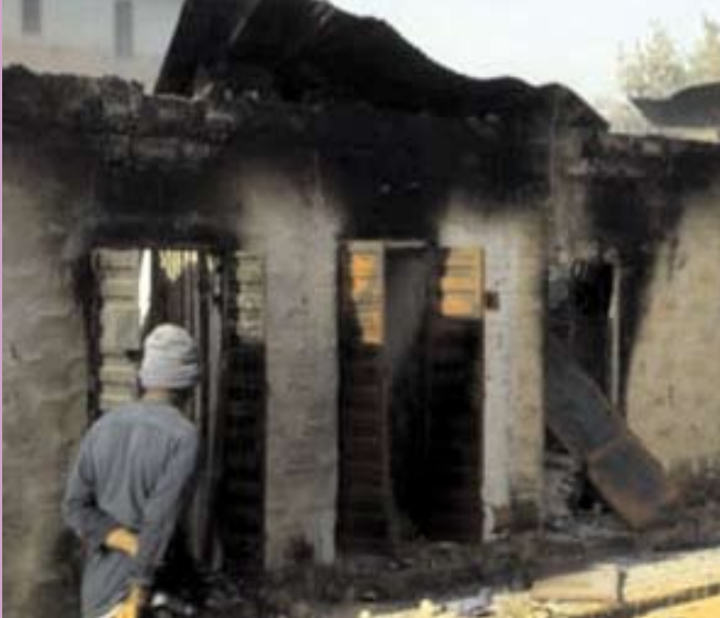
Home destroyed by rioting Muslims, Jos, Nigeria
