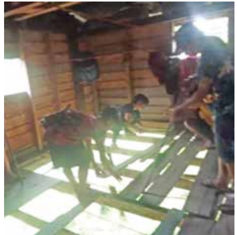
A widow-headed Christian family’s house being dismantled by order of the village authorities
