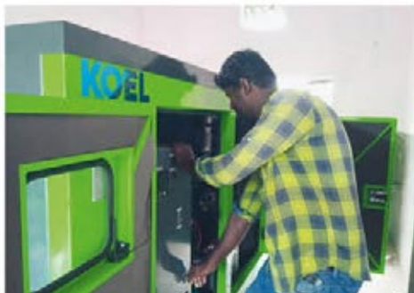
The new generator at Nav Jivan Hospital in Jharkhand state provides power for medical equipment as well as the onsite living quarters of hospital staff.
