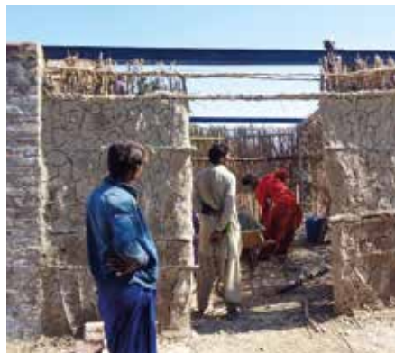
One of the new Barnabas-funded homes under construction, showing the brick-built pillars supporting the mud walls. Some of the iron girders that will support the mud roof are in place
