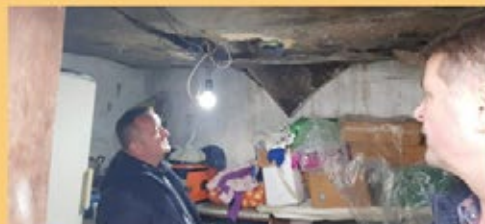
An Albanian pastor surveys earthquake damage to the ceiling in a Christian's home. While still recovering from the devastation of the double earthquake in November 2019, Albanian Christians were then struck with the coronavirus crisis
