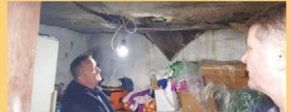
An Albanian pastor surveys earthquake damage to the ceiling in a Christian’s home. While still recovering from the devastation of the double earthquake in November 2019, Albanian Christians were then struck with the coronavirus crisis
